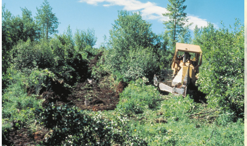
The C&H plough, mounted on a small bulldozer, is used to prepare sites for planting in areas of heavy vegetative competition.
