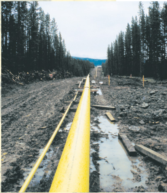
In the 1990s, about eighty kilometres of pipeline per year were constructed in the Hinton forest management area.
