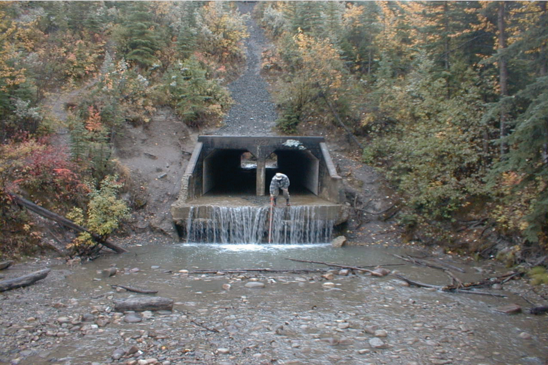
Exploring a waterfall at the outlet of the Canadian National Railways stream crossing prior to restoration work in 2003.
