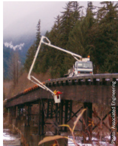
Two people using a snoop truck to check the structural integrity of the bridge.
