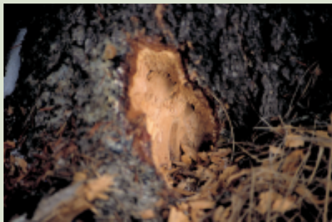
Sound wood is chipped away in the search for carpenter ants.
