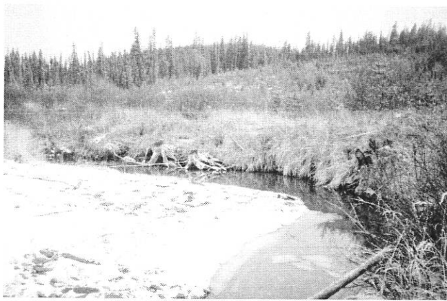
Figure 1. Upstream view of an eroding bank on the outside meander bend at Cross-section 12, in Upper Deerlick Creek, October 2001. Note the bank erosion in the vicinity of the stumps and lateral deformation of roots as potential indicators of the 1985 bank location.
